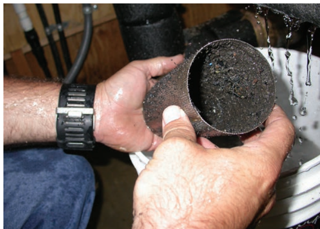
Photo 1: Ground loop and building systems must be properly flushed and purged of debris. Debris clogs system equipment and biological material contributes to a drop in water pH as it decays.
